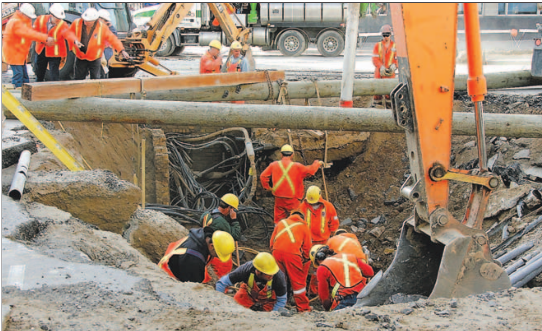
Crews from London Hydro clear debris from a giant sinkhole that opened early in the morning in the middle of a downtown intersection in London, Ont., yesterday. The street collapse, caused by a break in a water main, led to traffic backups and a power outage, closing much of the downtown area for the day.
